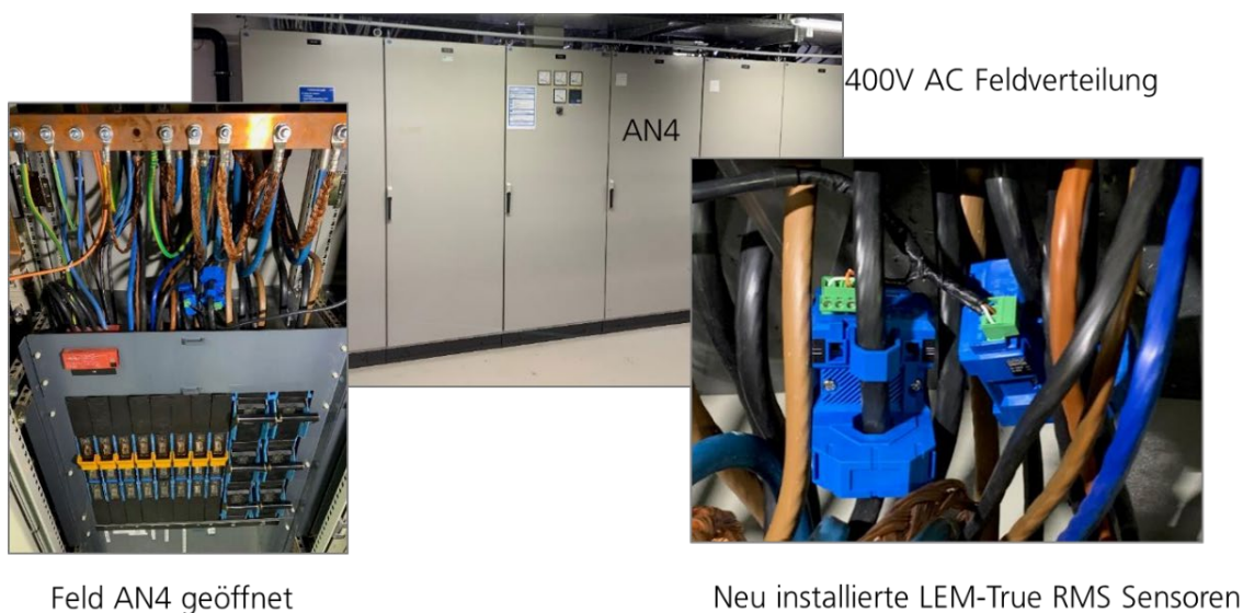
Figure 12: Current sensor installation on the process systems at the EMFT
